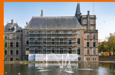
An extensive maintenance project, the Dutch historical Binnenhof is now being renovated to modernise its systems, welcome more visitors in the future and become more accessible for people with a disability.
