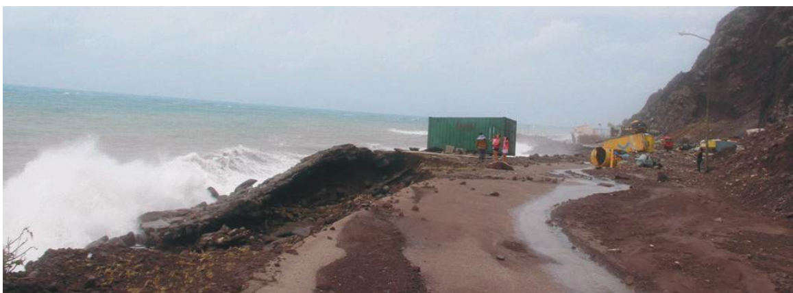
Figure 3.6 Landslides and debris blocked road towards Saba's Fort Bay Harbor, photo by Hazel Durand
