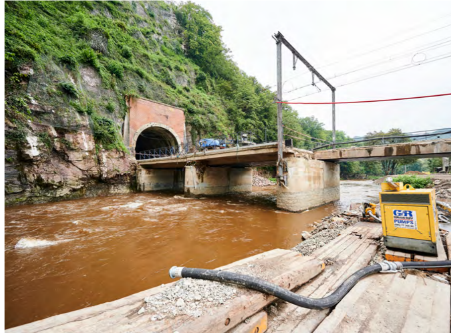
Damaged bridge during the floods in Belgium in July
