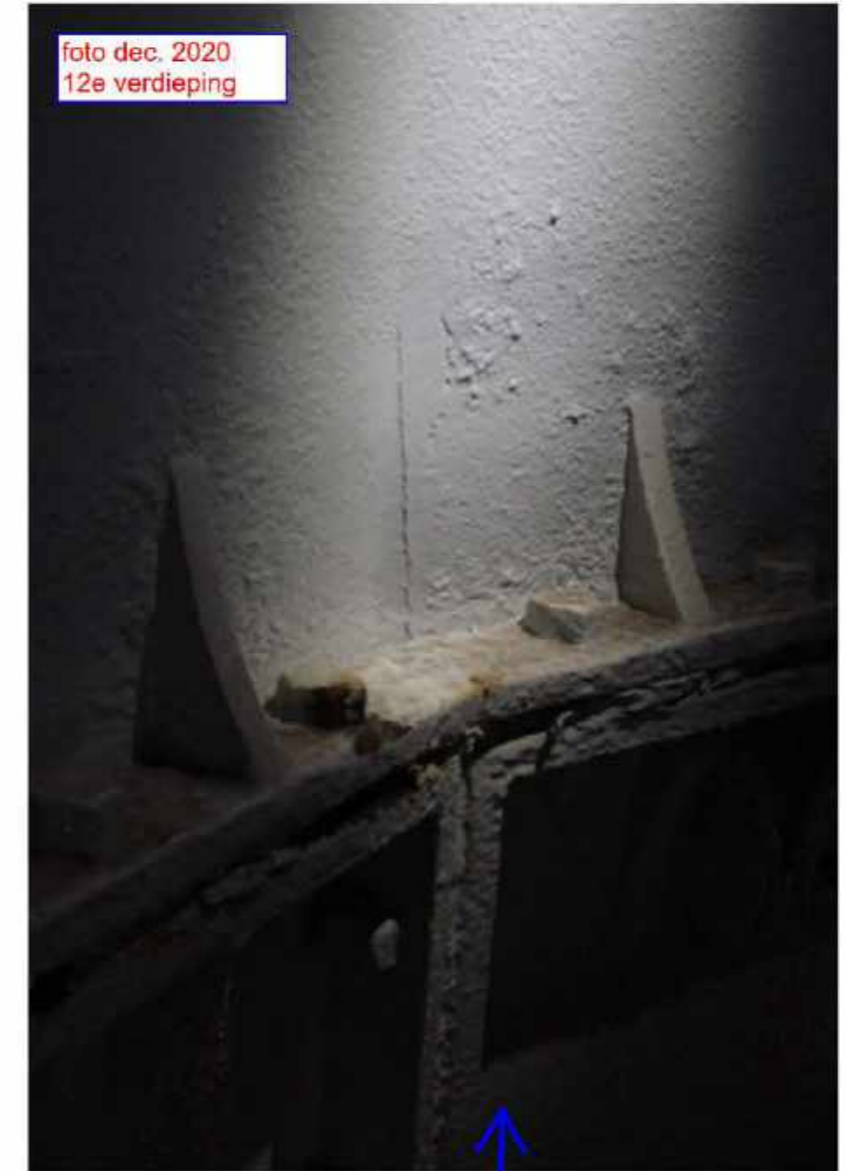
Verticale scheur in wand
