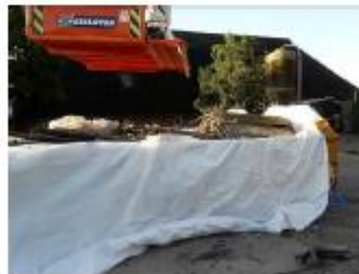
Foto: asbest in container
