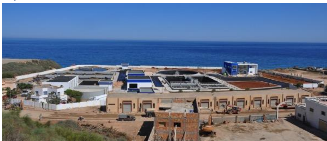
Figure 34: Al Houceima WWTP
