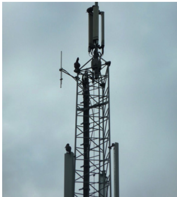
Illegale FM-antenne in mast mobiel netwerk
