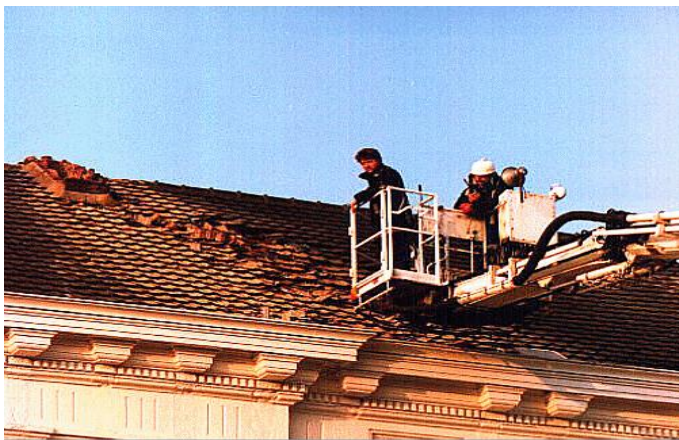
Figure 28 Roof tile connection failure during the Roermond earthquake, Netherlands 1992.
