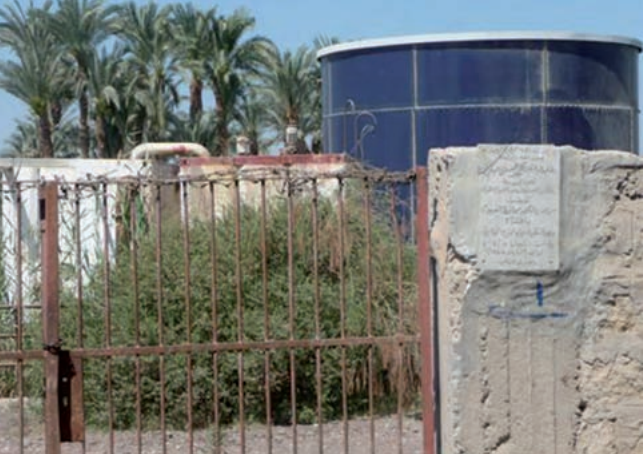
Compact water treatment unit
